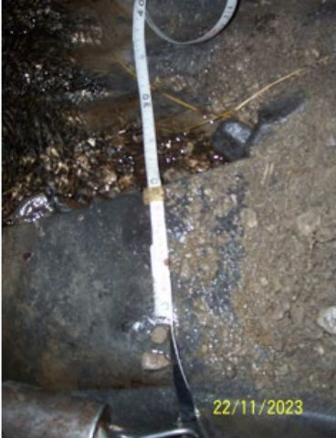
Culvert separation at floor Approx 300 mm
