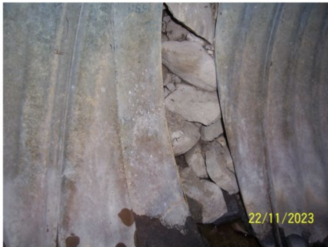
Culvert separation at the side wall
