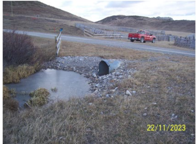
U/S profile Showing culvert end has heaved
